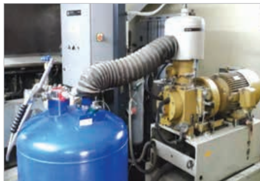
Figure 17 : Liquid Nitrogen Facility
